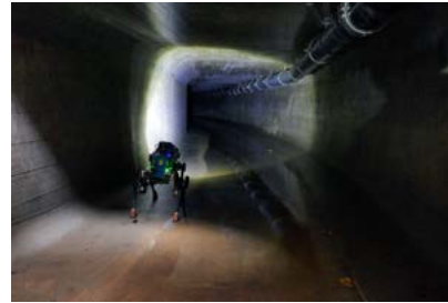
(c) Mission 2 in the second tunnel. Here the sewer is more curved and there is a large pipe suspended from the ceiling.
