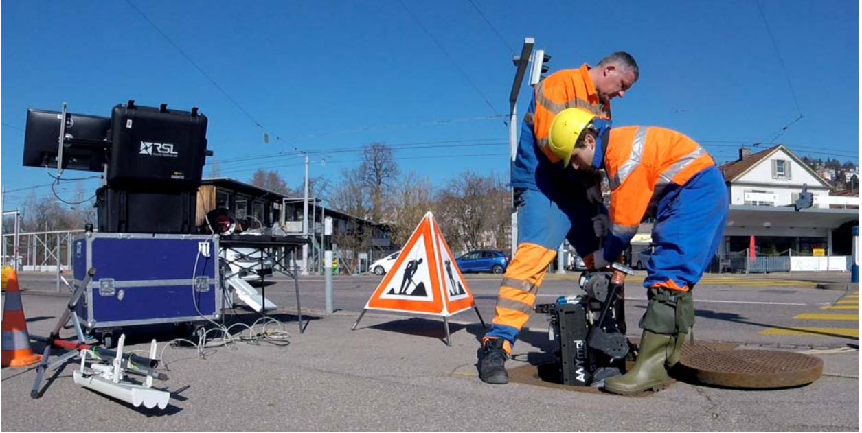
Figure 3: Depiction of the field test setup and the deployment of ANYmal into the sewer. The operator base station and warnings signs are visible in the background.
